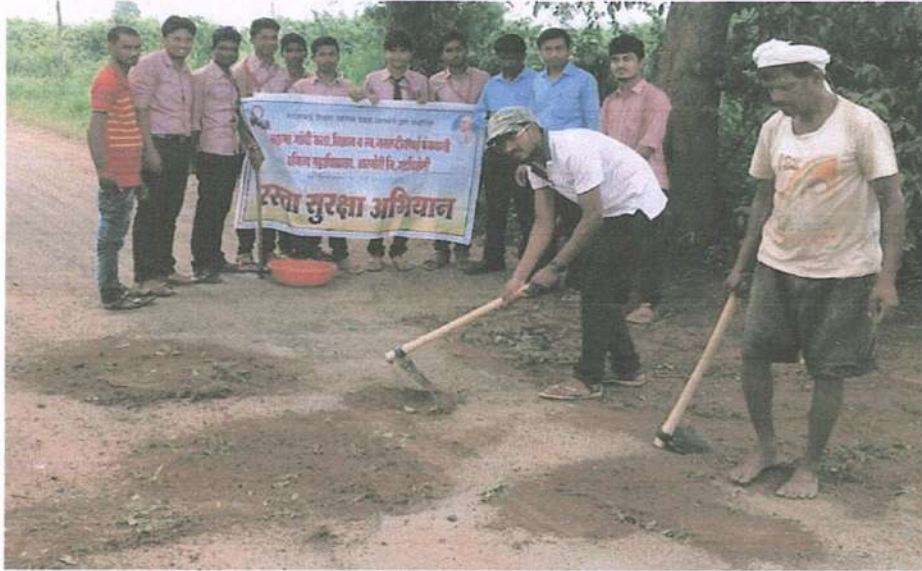
Path-hole filling under Road Safety Drive at adopted village Kasvi – 7 th October, 2016
